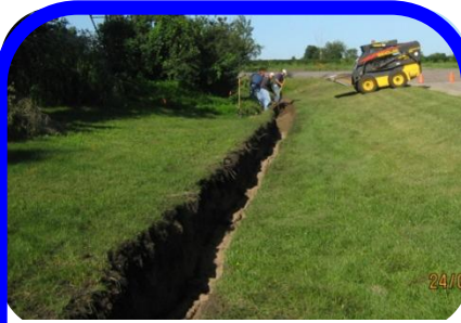
Soils were replaced in a 330 feet long trench to create 1,320 square feet of infiltration on the one side of the swale.
