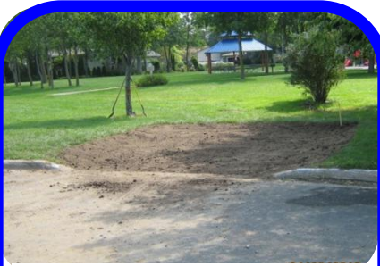
At three existing curb openings, poorly drained soils were replaced to create 250 square foot infiltration areas.
