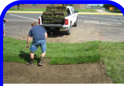
Turf sod installation was completed within backfill areas to avoid having exposed soils in the swale.
